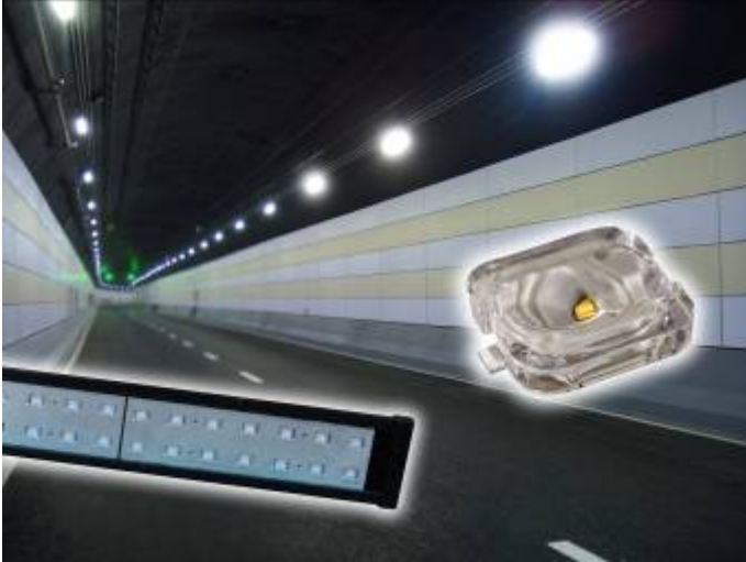
OSRAM's Golden DRAGON Oval Plus powered Zhonglong's tunnel lamps installed in Shanghai RenMin Road Tunnel
